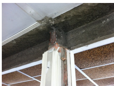
Figure 3. Example of concrete column in 7th floor, after removing the windows blinds.
