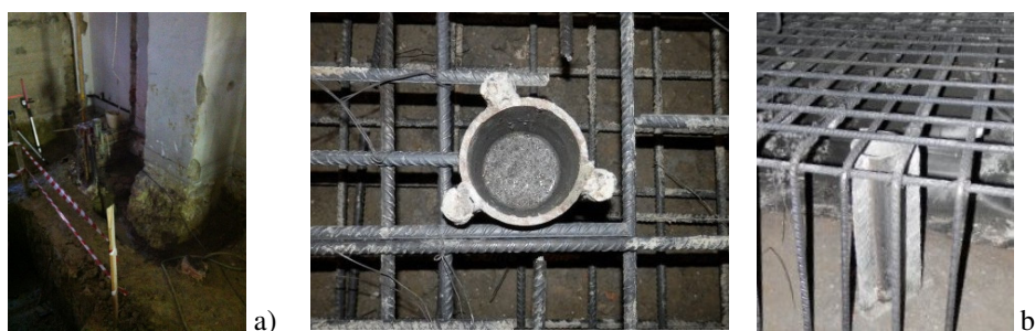
Figure 4. a) No foundation column; b) Micro pegs and mat foundation armour.
